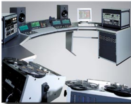
Example of a radio studio with an 18-fader Studer OnAir 2000 console, a broadcasting workstation running Studer DigiMedia, two Studer A807 tape recorders and additional equipment for DJ operation, planned and installed by Studer.
